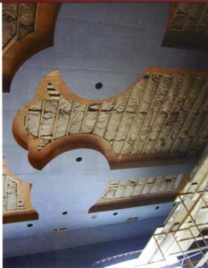
Multiple areas of a residential bathroom ceiling being prepared for installation of digitally printed fabric over acoustical material to reduce reverberation. PHOTO COURTESY SH! ACOUSTICS
